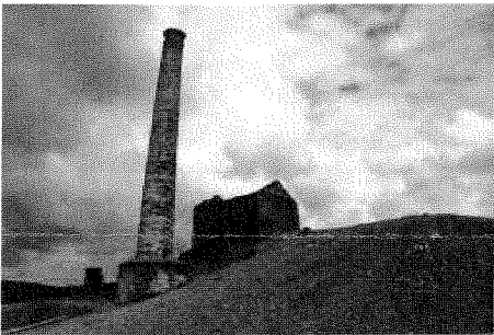
Beckwith's Mine at Foxdale is well known on the island for its leaning chimney.
